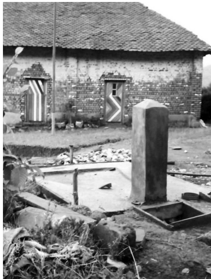
Drinking fountain during construction work, Kyuna primary school and Kisanga Institute, Kisanga
